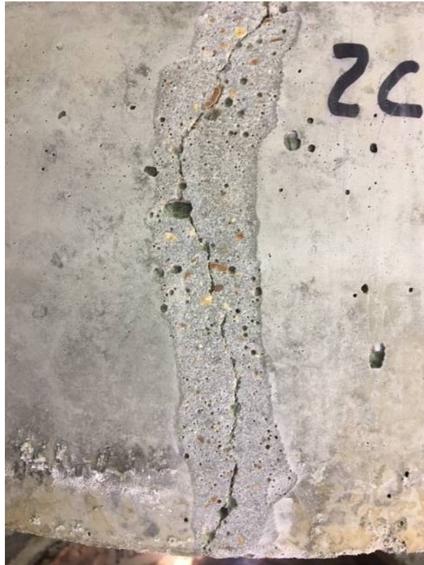
Figure 16. Surface Preparation of a Drying Shrinkage Crack (Mix 2, Ring C)
