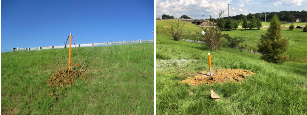
Figure 4.17 Inclinometer casing at Slope 2
